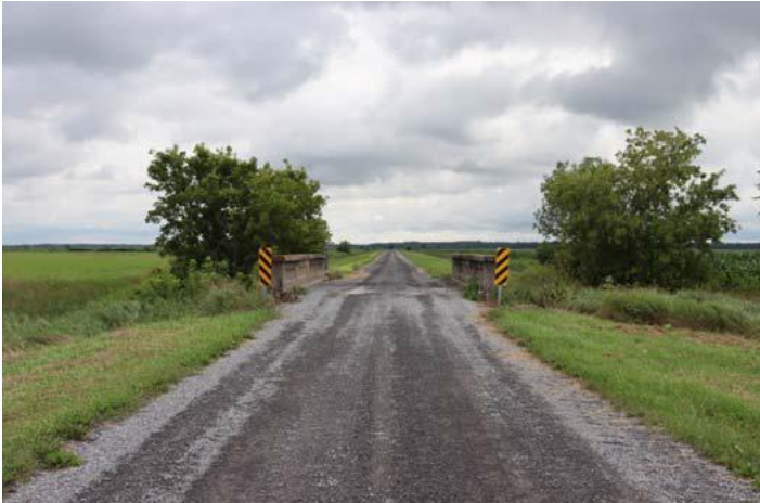
Very Poor Condition – BCI 42.7 – Concession 8, Paxton Creek Bridge
