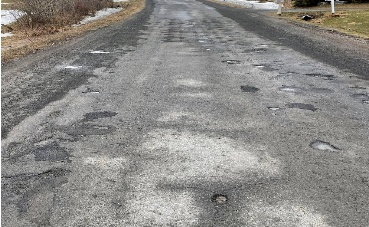
Very Poor Condition – Concession 19
